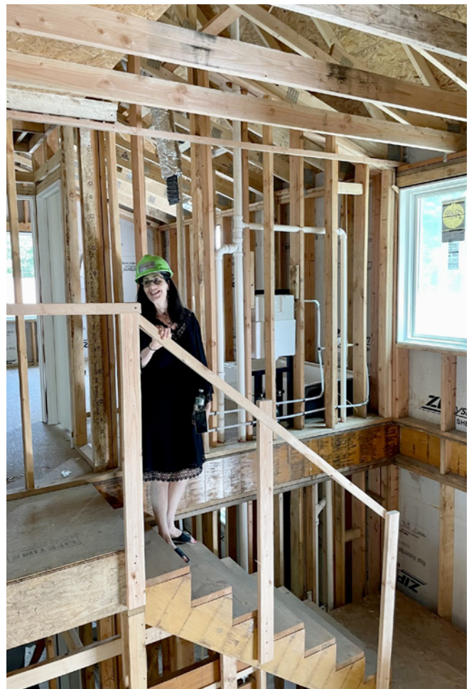
Allyx Schiavone, executive director of Friends Center for Children in New Haven, visits the site where Yale Architecture students are building new housing for her staff. ERICA E. PHILLIPS / CT MIRROR
